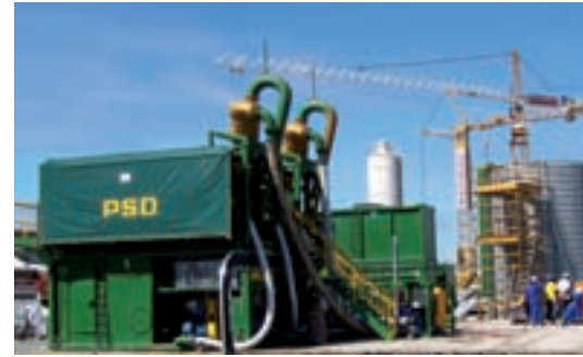
STP at Durban Harbour Tunnel
